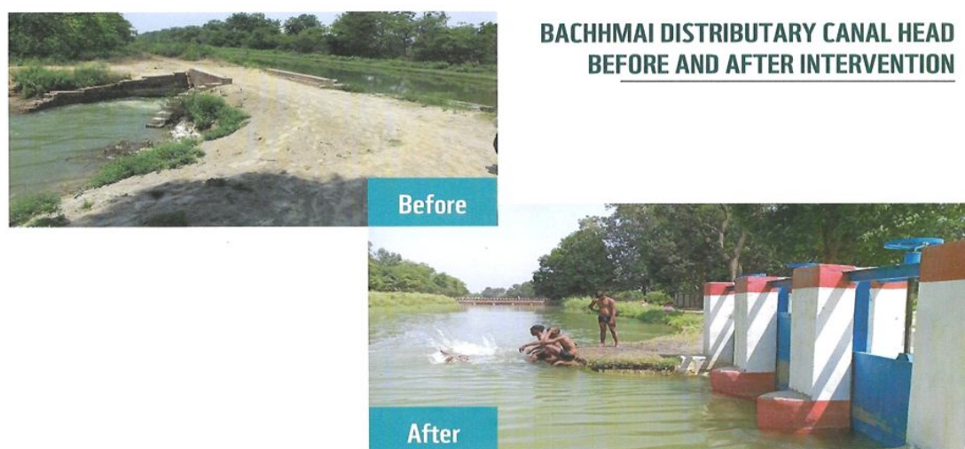
Figure-1 Head Regulator of Bachhmai distributary off-taking from Farrukhabad branch of LGC before and after project intervention
